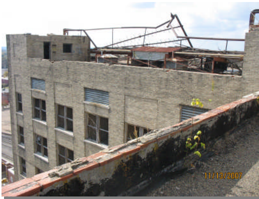
Façade in significant disrepair, vacant for 40 years.
